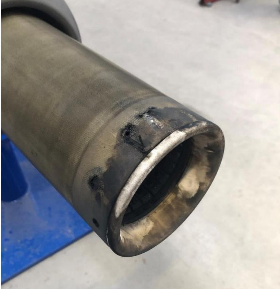
Figure 12 Puncture holes in the interrupter casing.
