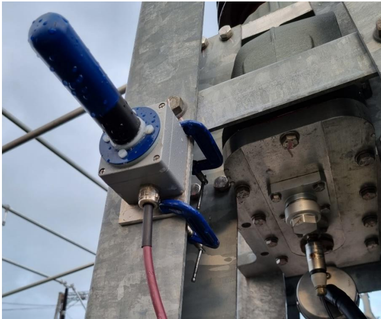
Figure 6 RF antenna clamped to the supporting structure of the blue phase interrupters.
