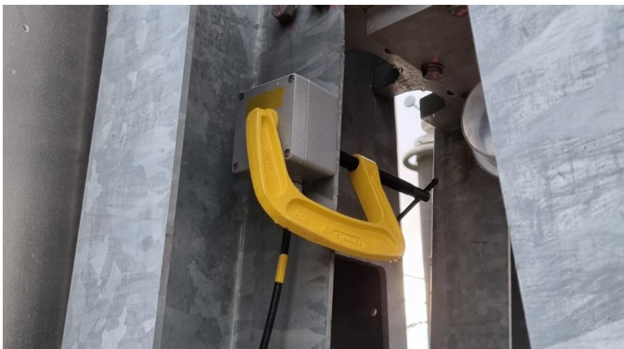
Figure 2 Vibration sensor in situ.
